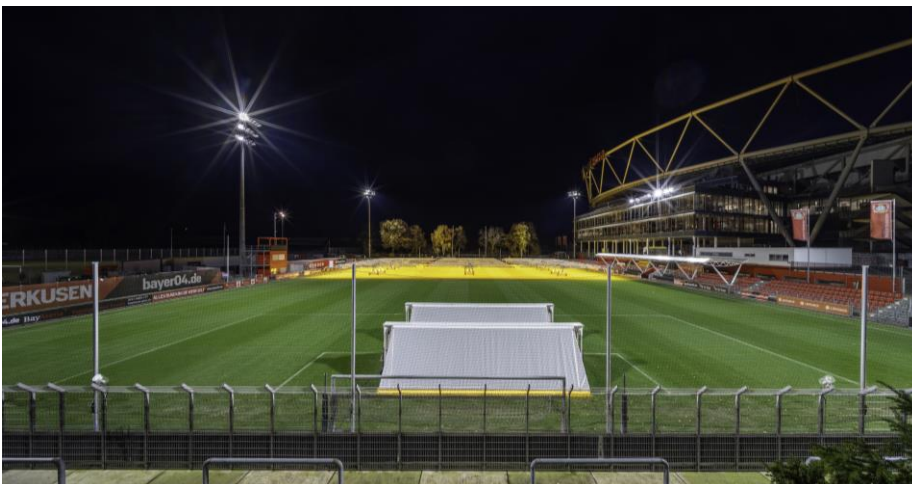
Field illumination inclusive new mast
